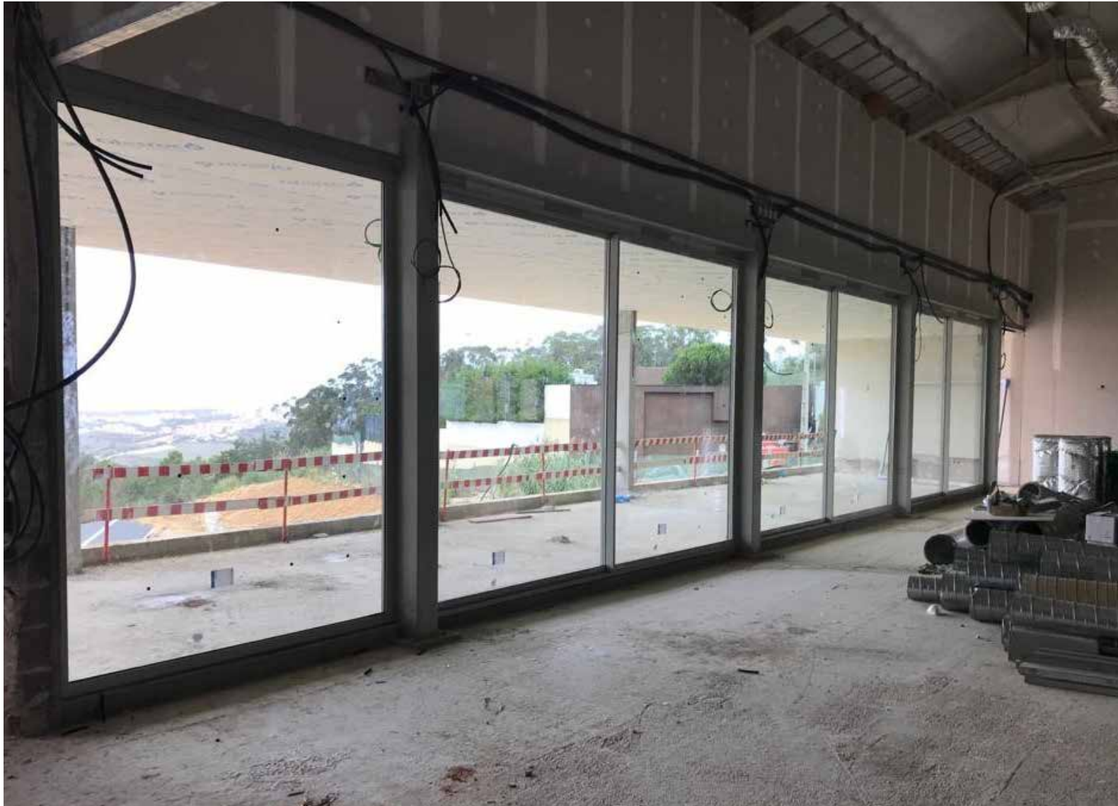
Work in Progress. 5 Star Hotel in Ericeira. Architecture by Tiago Silva Dias Arquitectos.
